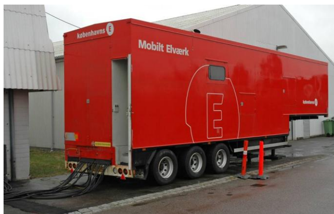
Exhibit 24: A mobile back-up generator participating in demonstration project about new sources for regulating power.
