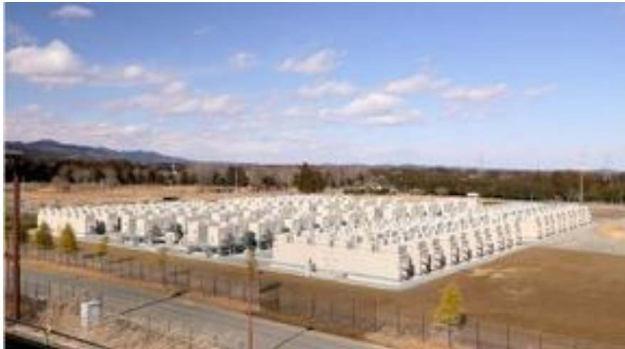
Figure 61: Picture of the 40 MW and 40 MWh energy storage system in Fukushima, Japan.
